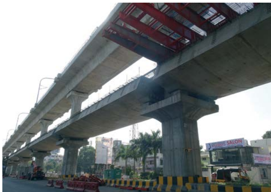
Investment in sustainable transport boosts the economy: New metro under construction in the Indian city of Nagpur in 2019.
