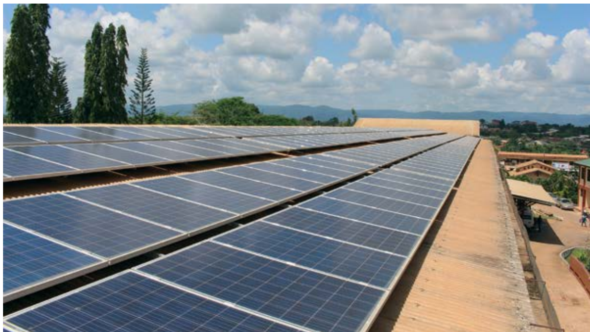
Solar modules at St. Dominic Catholic Hospital in Akwatia in the south of Ghana.
