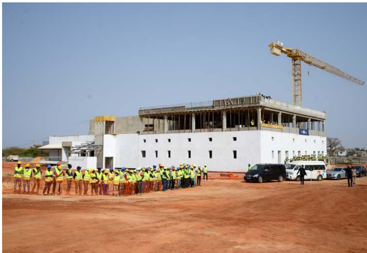
Construction of a vaccine-production plant supported by Germany and the EU by Biontech and the Institut Pasteur de Dakar in the Dakar region, 2022.
