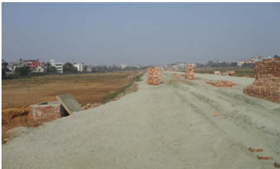
New transport infrastructure will have long-term impacts: road construction on the fringes of the Dhaka agglomeration in Bangladesh in 2017.
