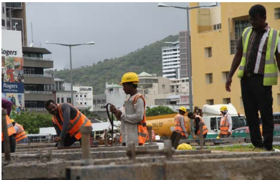
Building a light-rail transportation system is one of Mauritius' measures to curb emissions. Construction site of the Metro Express in Port Louis, the capital city.
