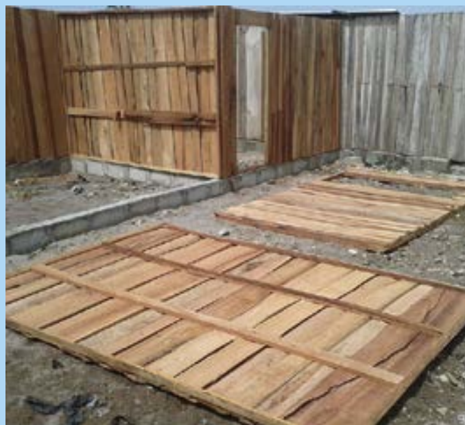
The design of the simple timber units is based on a modular system.
